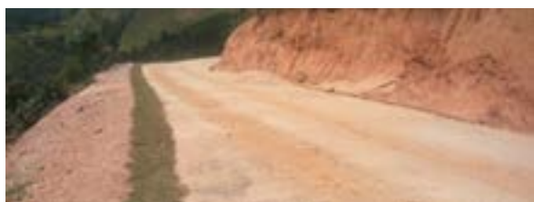
Concrete paving at high slopes ensure mobility during the rainy season with greening to avoid erosion. Photo by Dieudonne Niyigena
