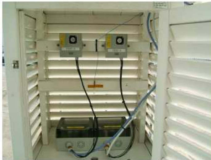
Example of Installation of PM Sensor and Interface Board in Thermometer Shelter
